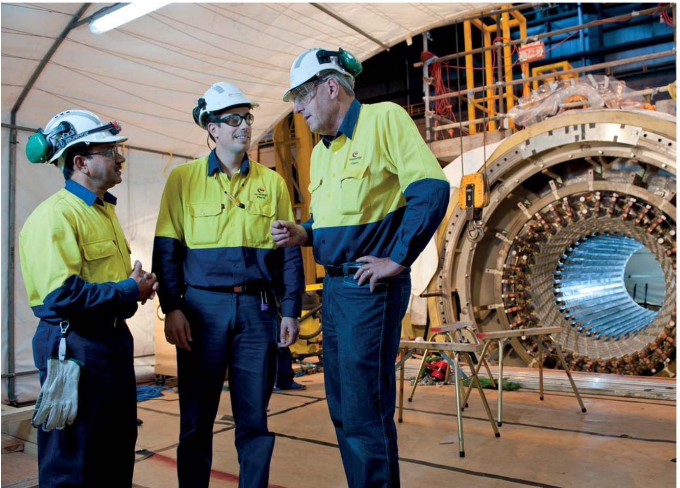
Gary Campbell, General Manager Production (right) inspects the Callide Power Station Unit B1 generator rewind with Dev Sharma and Pierre Michaud.
